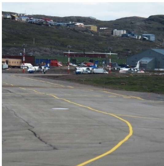
Figure 1-2 Ground settlement due to freezing-thawing action on the taxiway of Iqaluit International Airport (Natural Resources Canada 2017).
